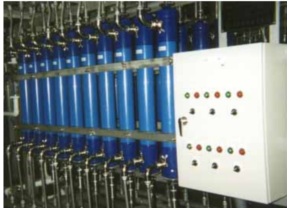
Drinking water production plant
