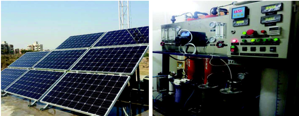
Fig. 3. Pilot scale Reverse Osmosis (RO) Plant at National University of Sciences and Technology (NUST), Islamabad, Pakistan
