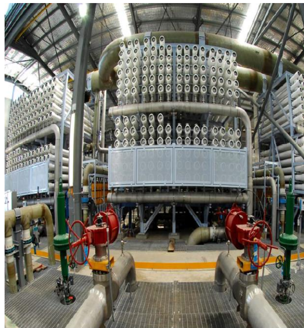
Fig 2.3: Perth SWRO plant (Hoang et al., 2009)
