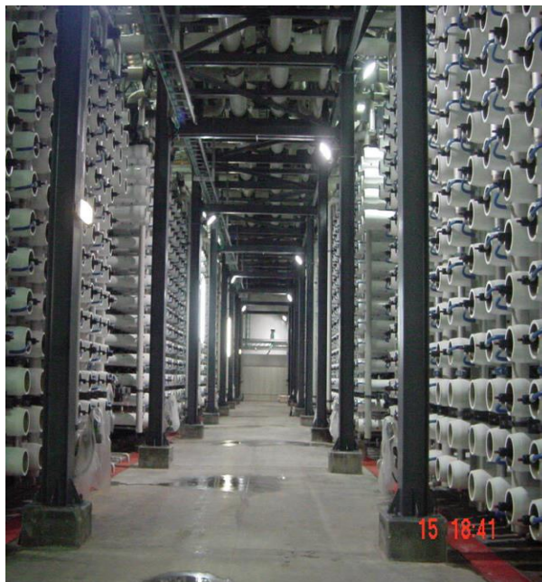
Fig 2.2: Ashkelon SWRO plant (Goichon, 2007)
